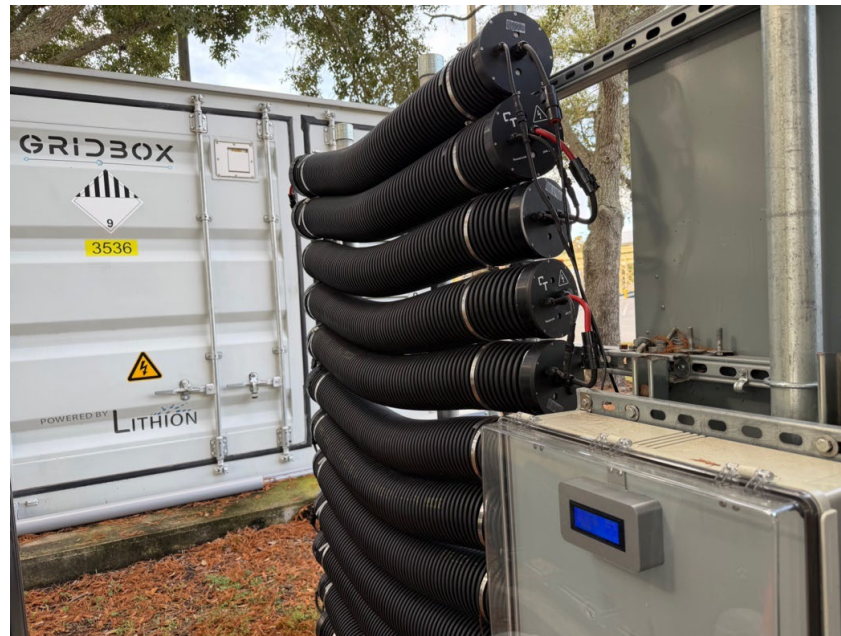
Fig. 11. System comprising 36 C-Link modules. System specs: 3.6F, 720V, 302 kW, 0.26 kWh
