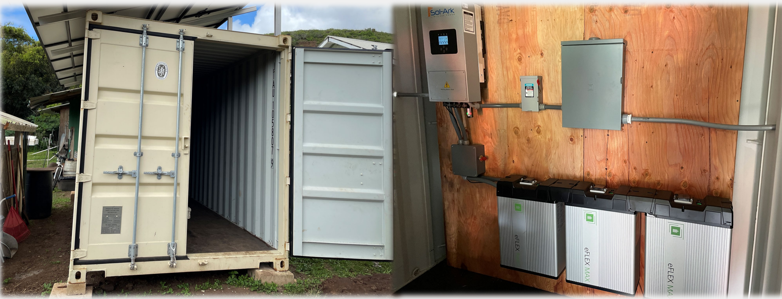
Fig. 2. Containerized Battery Energy Storage Installation
