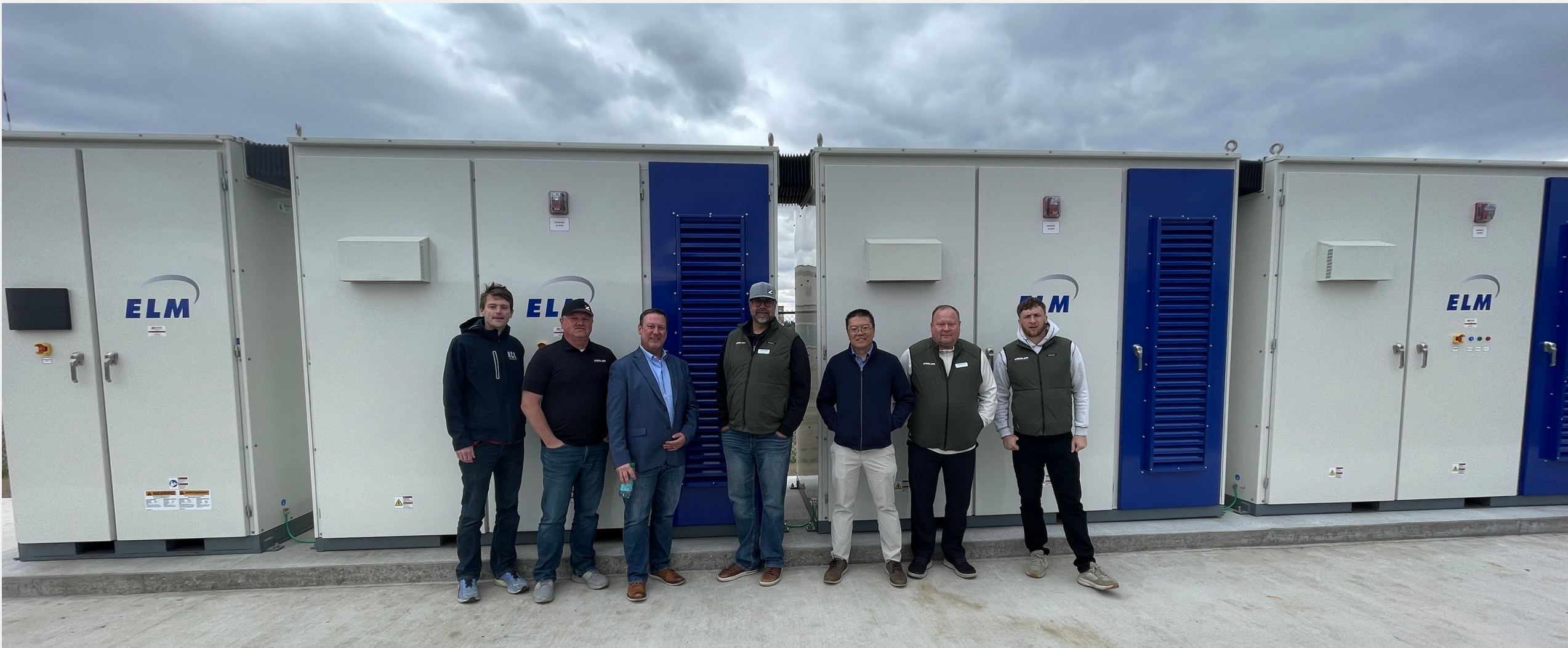
Fig. 1. Battery Energy Storage System at Pine Point School
