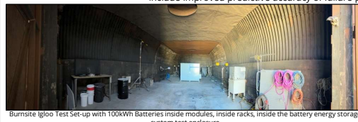
Burnsite Igloo Test Set-up with 100kWh Batteries inside modules, inside racks, inside the battery energy storage system test enclosure
